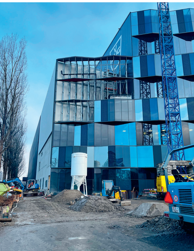
Installation of power facilities for the Multi Energy Hub into the existing warehouse building, “ZUGgate”
